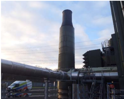
Felindre outer exhaust stack
