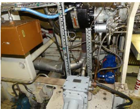
Kings Lynn gas generator showing stagnant areas below the engine that required additional ducting
