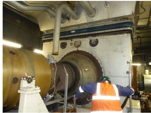
Power turbine/exhaust volutes lose internal lagging over time and cause overheating inside the cab
